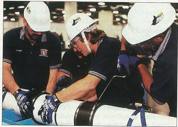
The St. Petersburg Devil Ray Claimers (Florida Water Environment Association) adeptly repair an in-service collections pipe during the Collections event.
